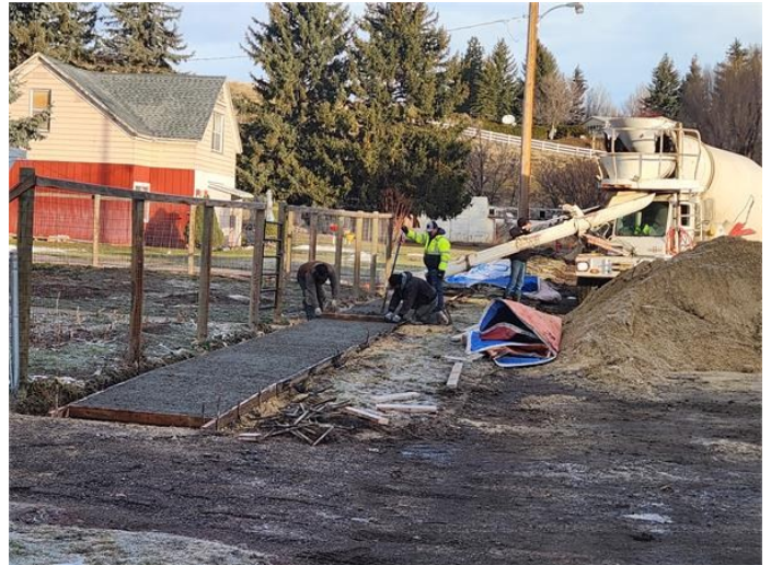
Subject: Concrete placement via truck and chute on West Street looking North.
